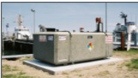
Marina Fueling Systems
