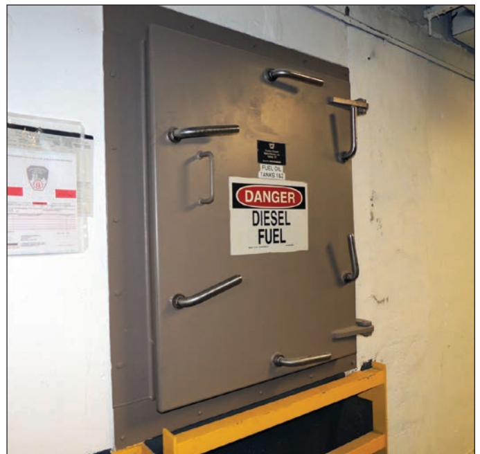
Figure 1: Fuel pump protected by watertight enclosure and "submarine doors" in Manhattan high-rise (top); 13,350-gallon fuel tank in a Manhattan high-rise protected by a similar method (bottom)
