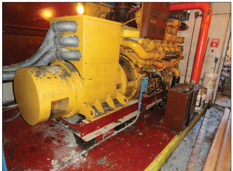
Figure 6: Emergency generator in a basement that was completely inundated during flooding from Hurricane Sandy (Long Beach, NY)
