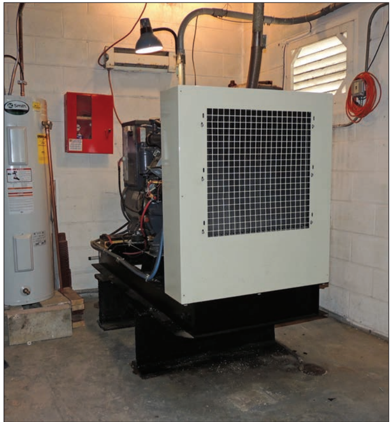
Figure 5: Emergency generator in a ground-level mechanical room that was inundated by 18–20 inches of water during Hurricane Sandy flooding. The generator was able to continue functioning because it was elevated approximately 20 inches (Ship Bottom, NJ).
