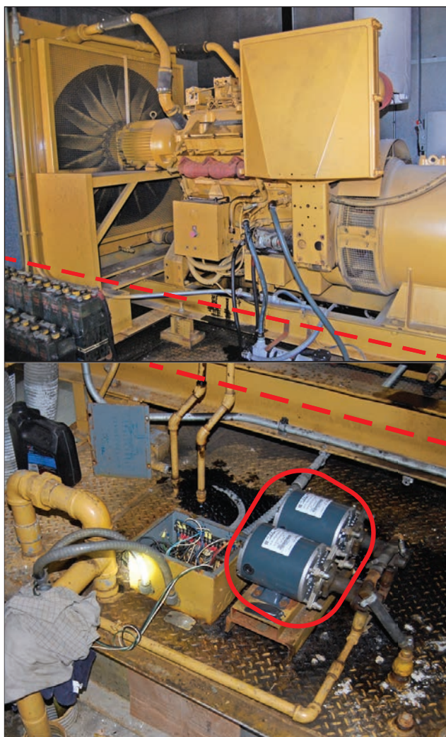
Figure 2: Unelevated fuel pumps and controls were flooded when floodwater reached the high water mark shown by the red line, causing the emergency power generator to fail (top). New pumps, located on the back side of the unit, were installed but not elevated to reduce vulnerability to flooding (bottom). (Long Beach, NY)
