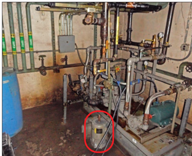
Figure 1: Hospital fuel oil pump (red circle) was flooded, resulting in failure of the emergency generator (Manhattan, NY)
